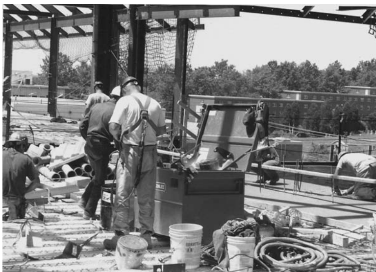
FIGURE 25.16 Poor housekeeping impedes travel and presents falling hazards.
